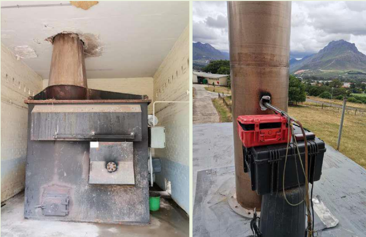
Images 1 and 2: In-stack monitoring for cremator's annual stack emission sampling
